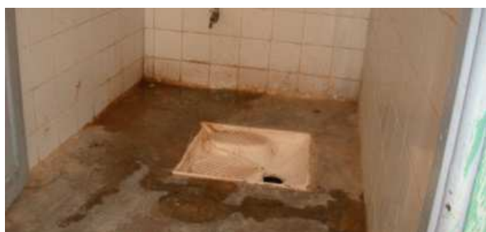
Figure 6: Latrine simple au Maroc (source: M. Wauthelet, 2012).
